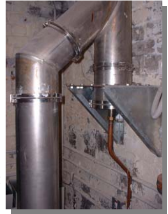
Gas Condensing Boiler
